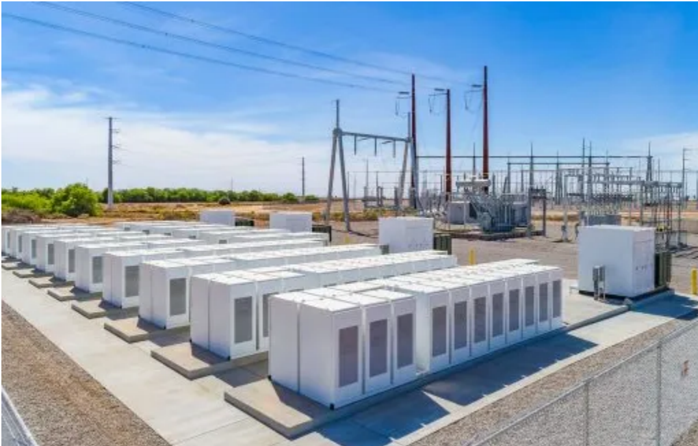
Figure14: Utility Scale Battery Storage System
